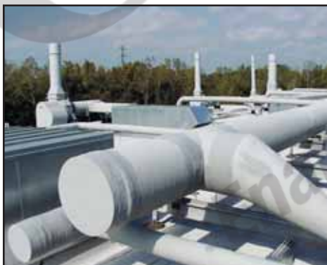
Methacrylate-silanes couple fiberglass to unsaturated polyester in corrosion resistant rooftop ductwork at Gelest, Inc.
